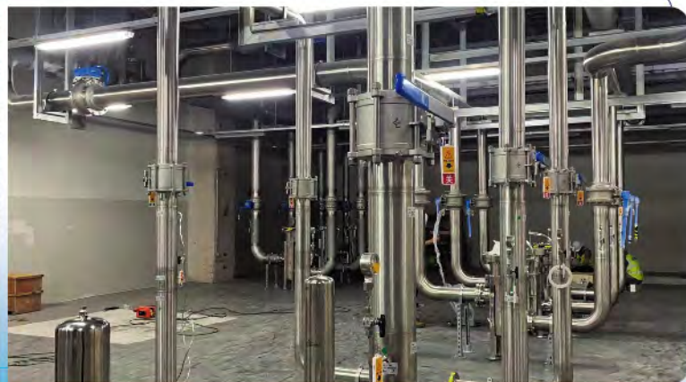
Bulk Gas System
