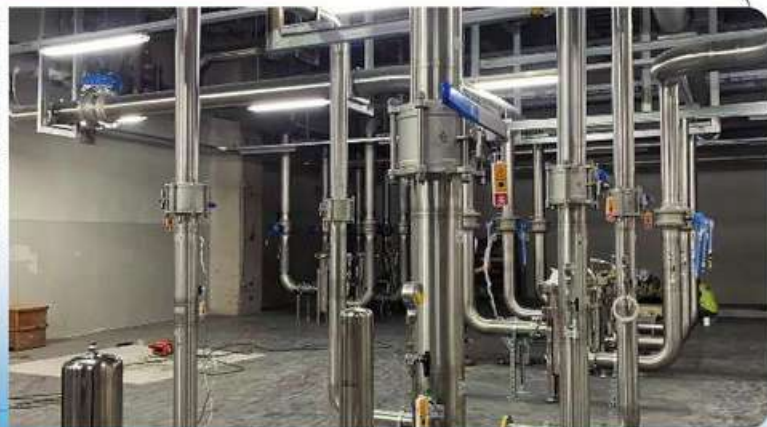
Bulk Gas System
