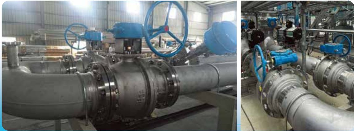
Bulk Gas System
