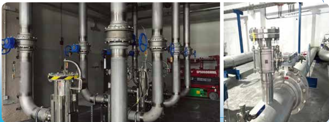
Bulk Gas System
