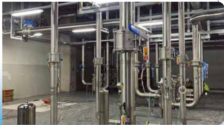
Bulk Gas System
