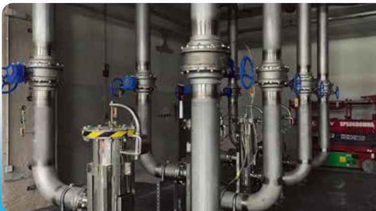
Bulk Gas System
