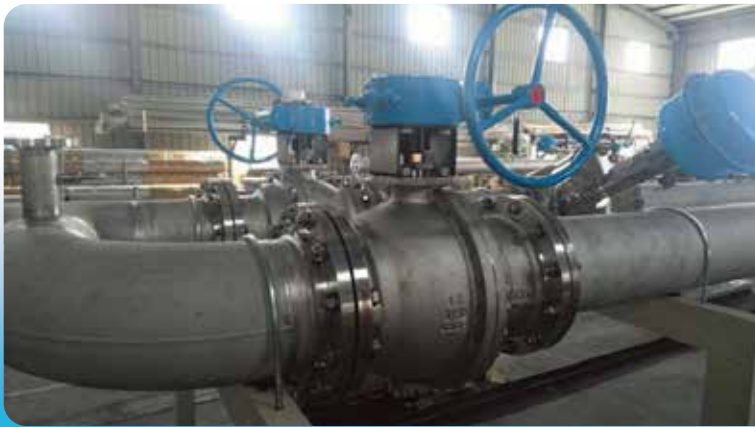
Bulk Gas System
