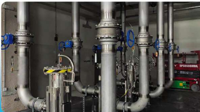
Buk Gas System
